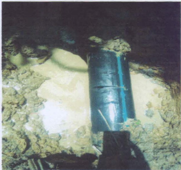
Picture showing spill point (Hack Saw Cut)
